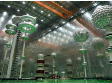
Securing World-Class High-Voltage, High-Power Testing Capabilities (Ranked 2nd globally)
